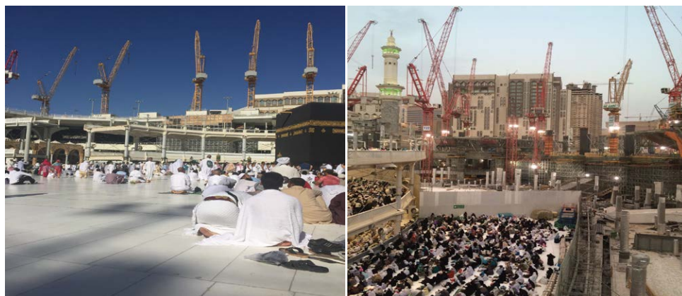
Fig. 3.2. Cranes at the 2015 Hajj festival, one of which collapsed. (Source: Razaq Raj)
